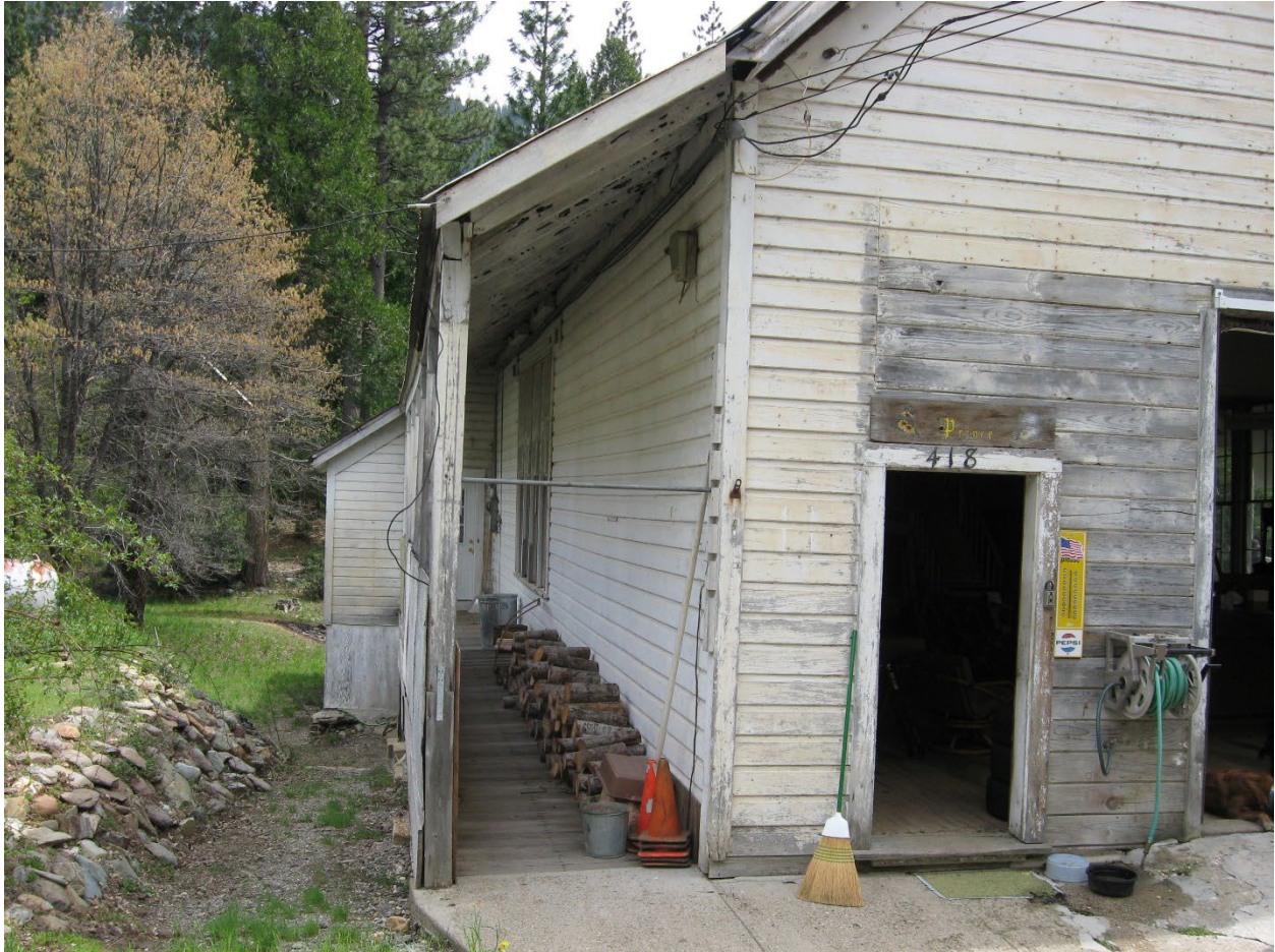
North façade and east porch prior to rehabilitation work after 2009 (Photo: Nora Prince collection)
